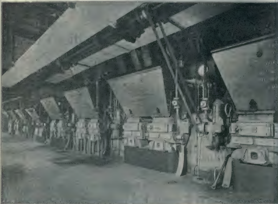
PHOTO OF A RANGE OF LANCASHIRE BOILERS. Fitted with the “Koker” Stoker and “Meldrum” Draught. Twenty-two Boilers have been fitted for this firm.
